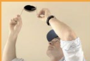
L section of wire frame clears the underside of the ceiling and fits into place – excess is removed
