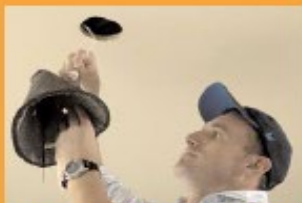
Wiring loom threaded through cover
